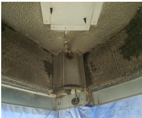
System cooling and heating equipment heat exchanger
