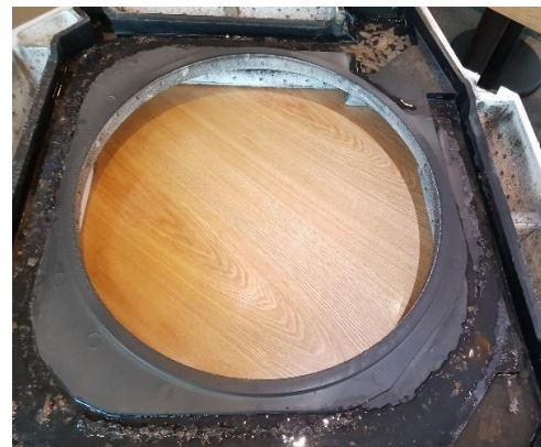
The drain plate Cooling & Heating system
